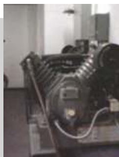
Air Compressor – Full Visible
